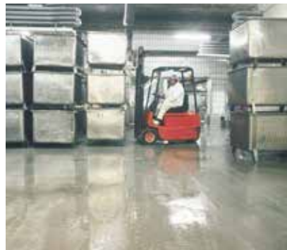
Densitop® in a cold storage warehouse.
